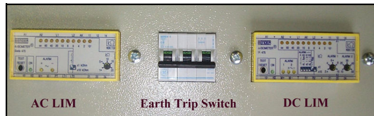
Figure. 1.4 AC and DC Line Insulation Monitors
