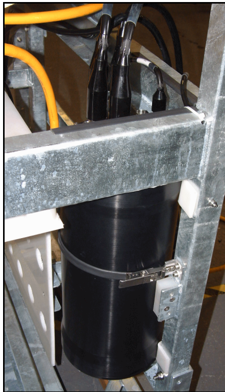
Figure. 5.1 Electronics Pod TMSEPM-2D
